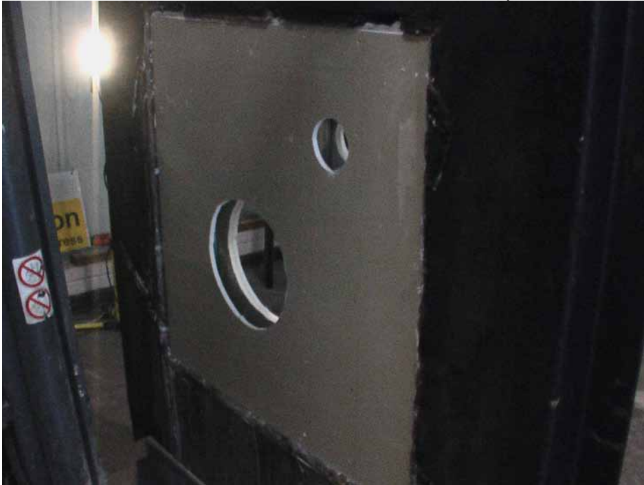
FTP 3 Wall with double skin inside and one outside prior to the last external skin.
