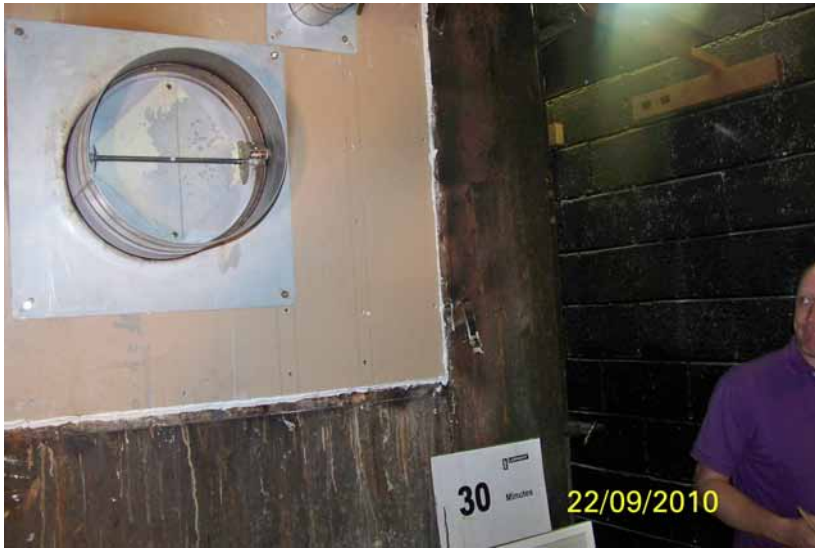
FTP13 Fire test after 30 min's
